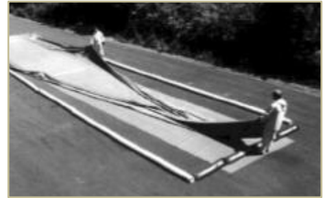
A portable containment pad can be constructed to collect wastewater from power washing. *Photo courtesy of GMC Delco Cleaning Systems.
