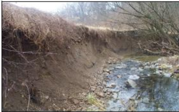
Before: This Mill Creek tributary was cutting into a federally funded water quality basin
