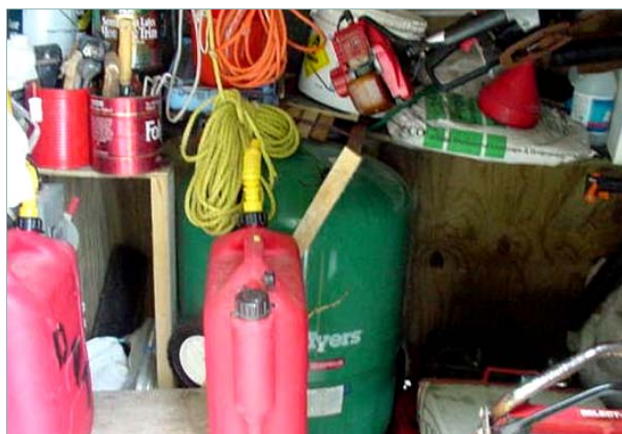
Figure 4. Clutter near drinking water equipment
